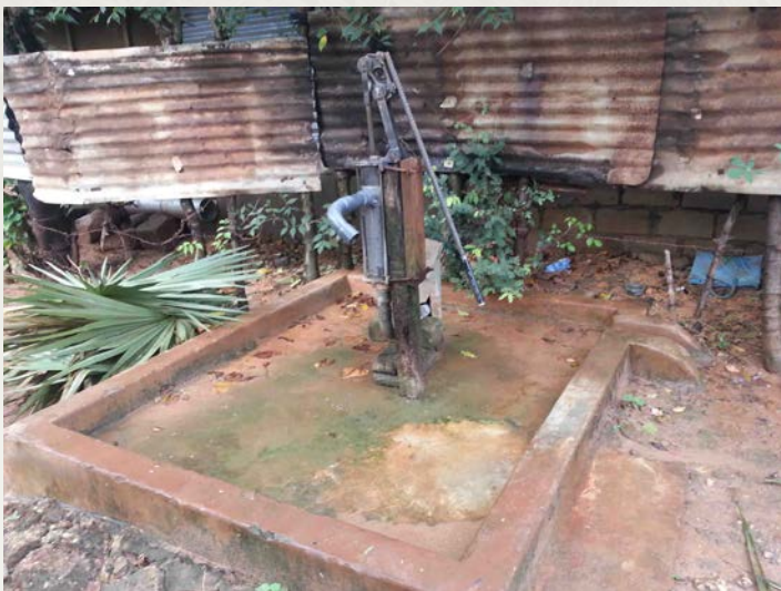
Faucet for the use of the residents of Camp Sabapathippillai.
