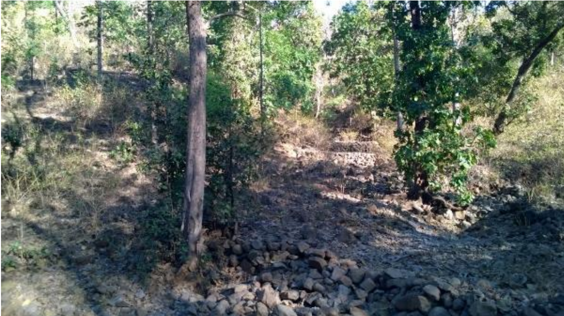
Picture 20 – Loose boulder check dams in series in Parasda village, Bhaura range, Betul
